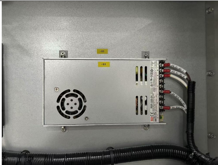
Photo 17- 24V Power supply
