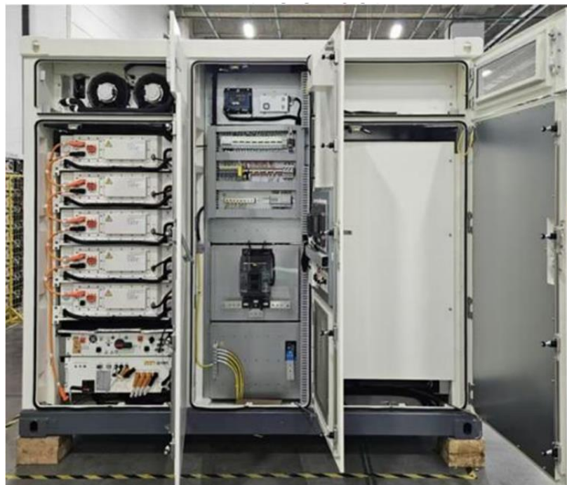
Photo 8-Internal view 1 front side (CESS466-250-01D)
