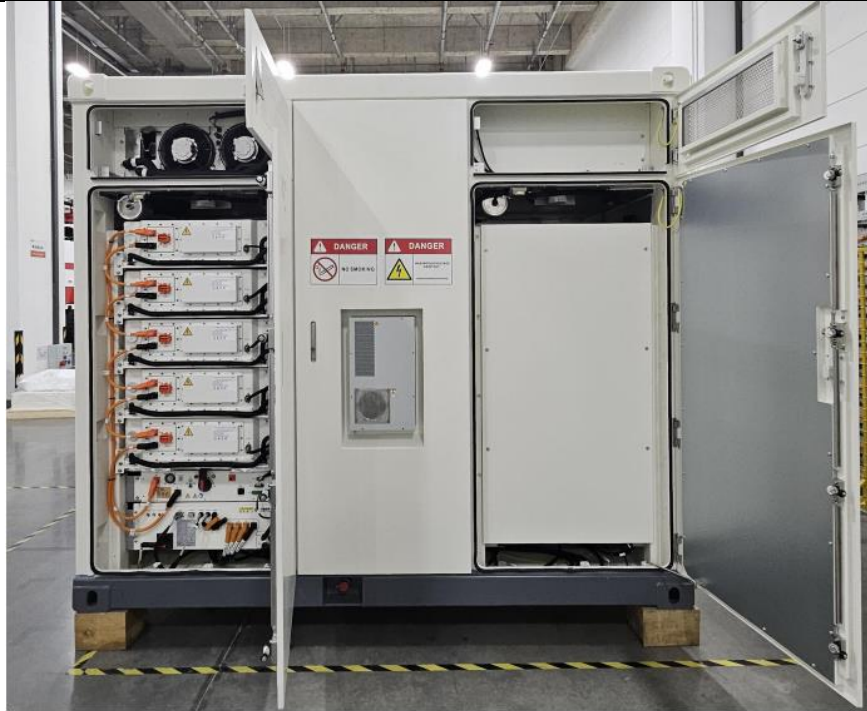
Photo 9-Internal view 2 back side (CESS466-250-01D)
