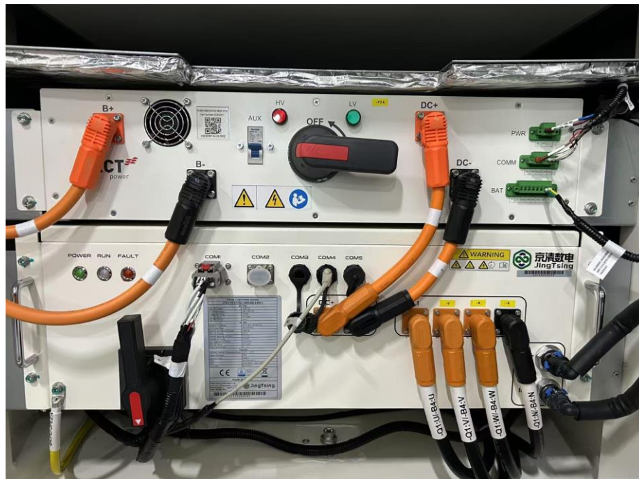
Photo 12-Switch gear and PCS module
