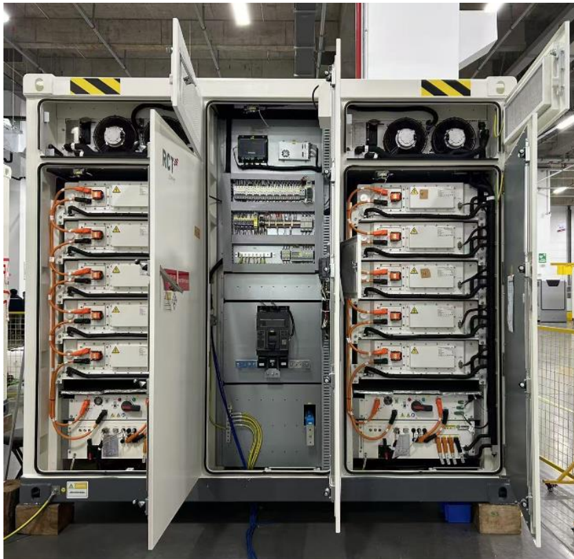
Photo 6-Internal view 1 front side(CESS699-375-01D)
