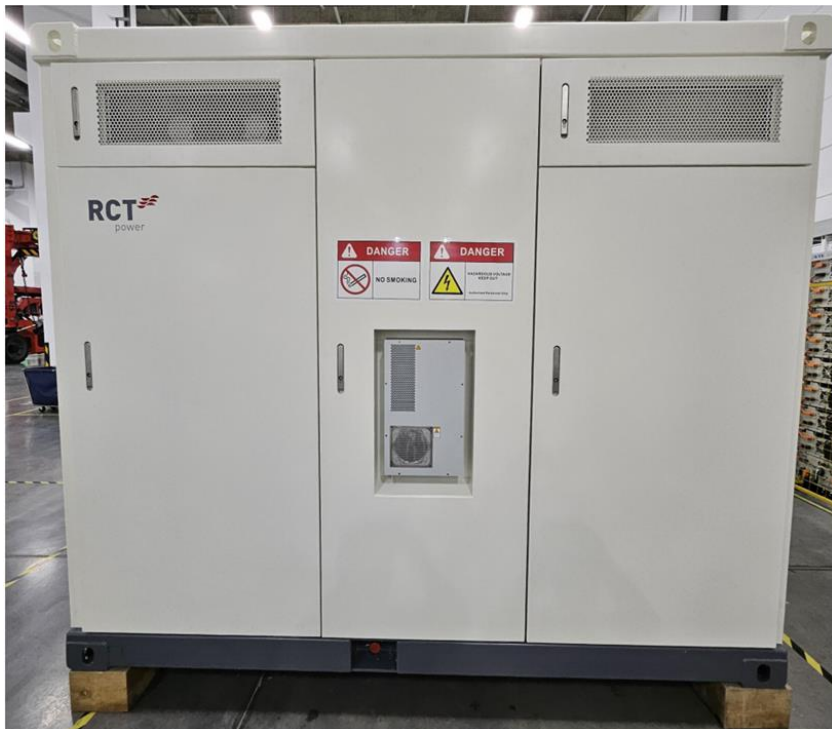
Photo 2-Back view of CESS932-500-01D
