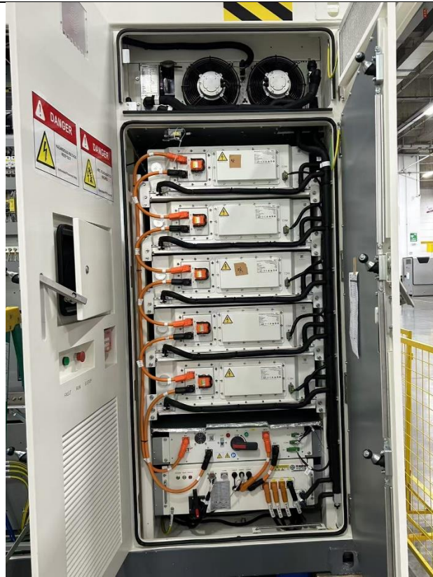
Photo 11- Battery rack with PCS
