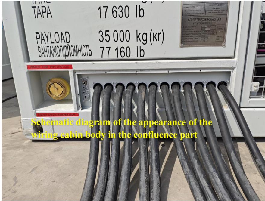
Figure 5-9 Schematic diagram of the appearance of the junction compartment of the confluence part
