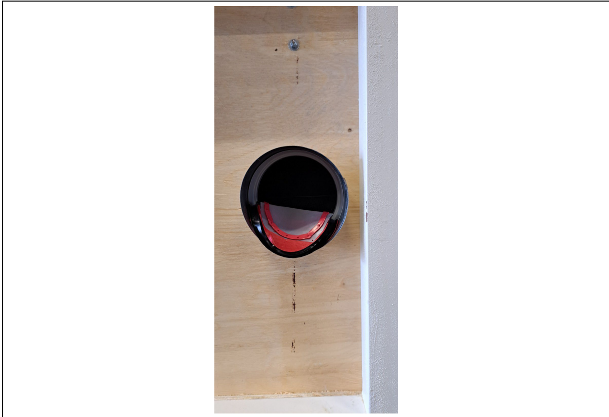
Photo C. 9: Damper A (exposed side)
