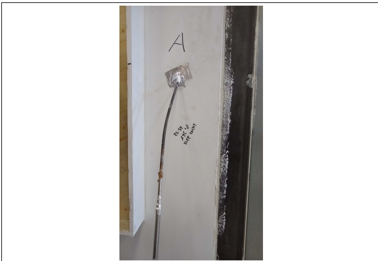
Photo C. 6: Closing time damper B
