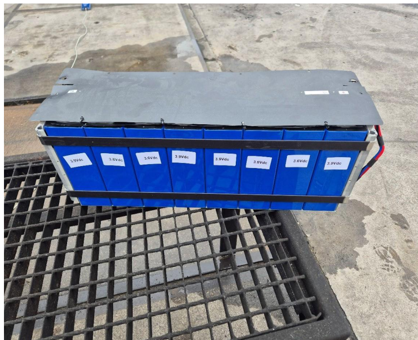
Figure 1 - Overview of battery pack.
