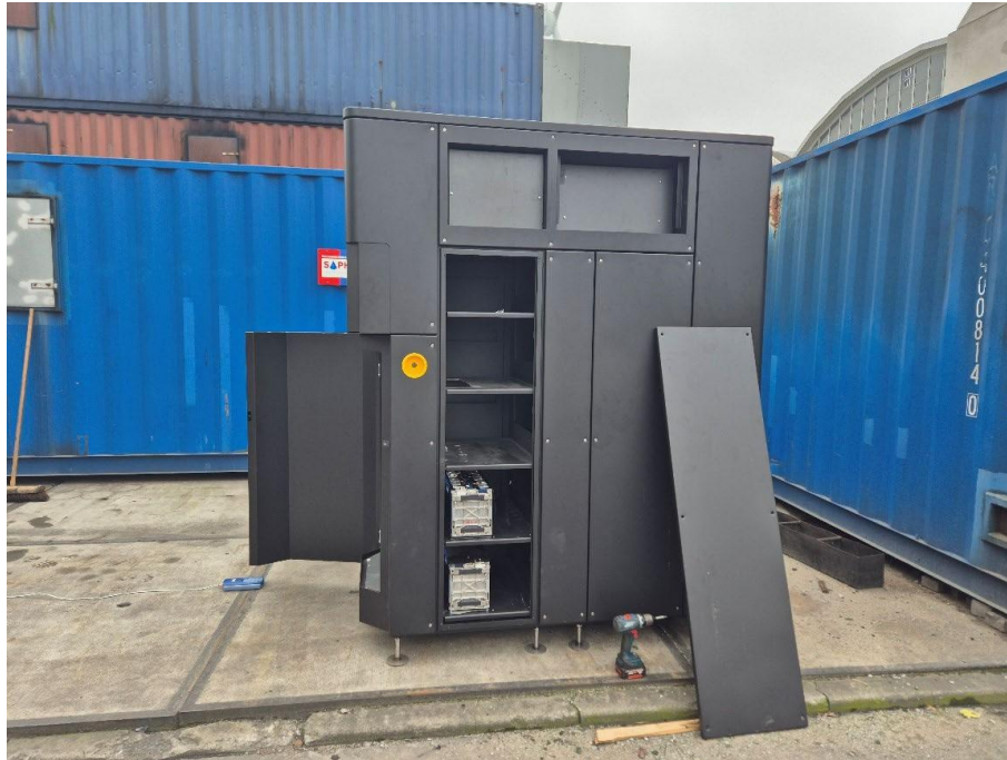
Figure 2 – Cabinet prepared for propagation test.
